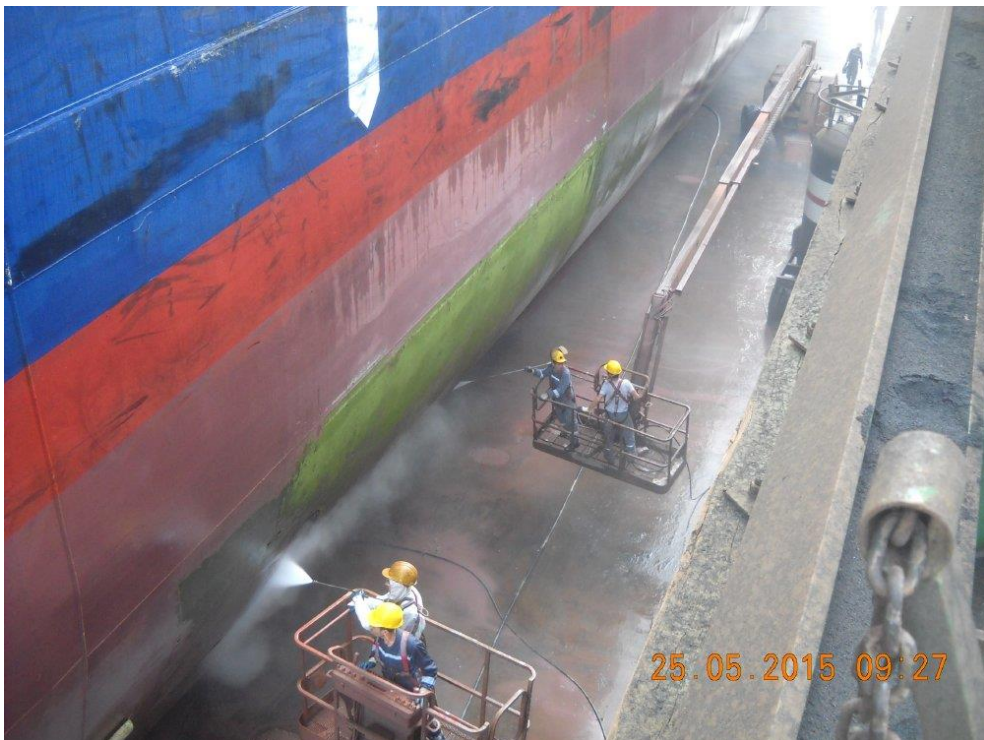
Figure 4.43. VESSEL 5, 2015 Dry-dock, photo of hull condition, during high pressure water washing
