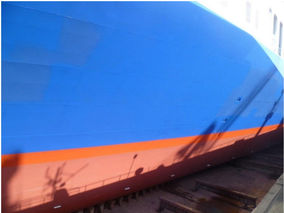
Figure 4.49. VESSEL 6, 2013 Dry-dock, photo of hull condition, after 1 st type self-polishing coating application
