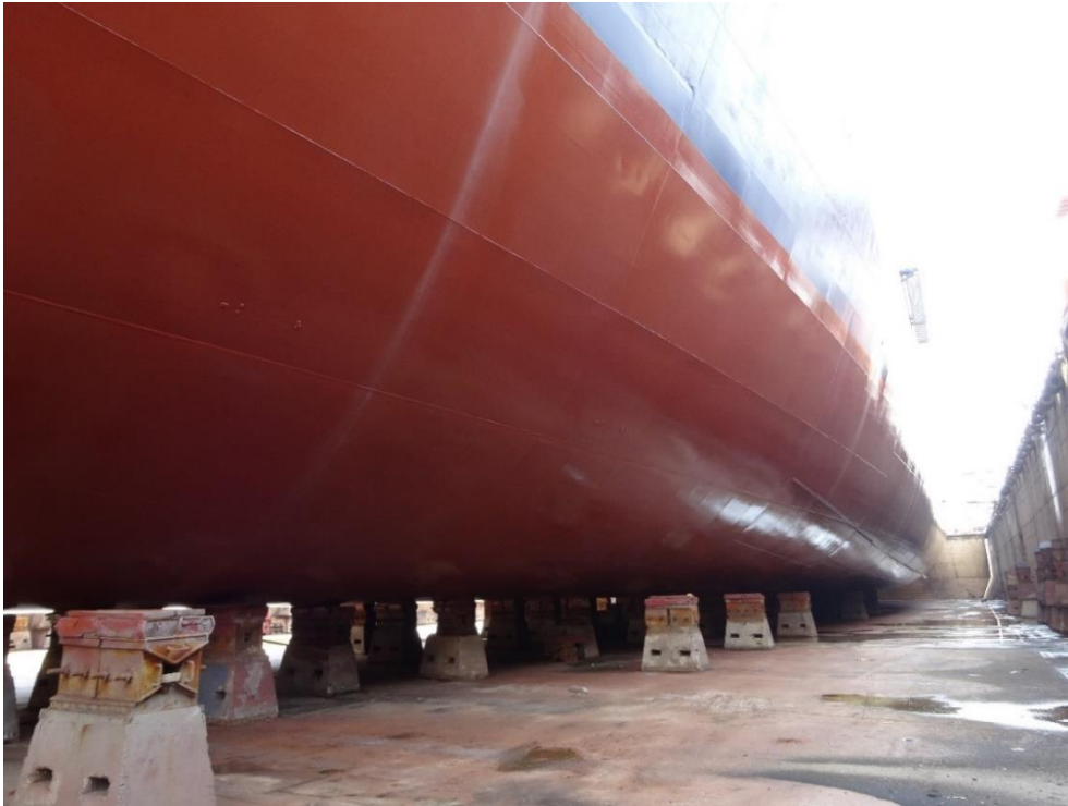
Figure 4.14. VESSEL 2, 2014 Dry-dock, photo of hull condition, condition after 1 st type foul release coating application
