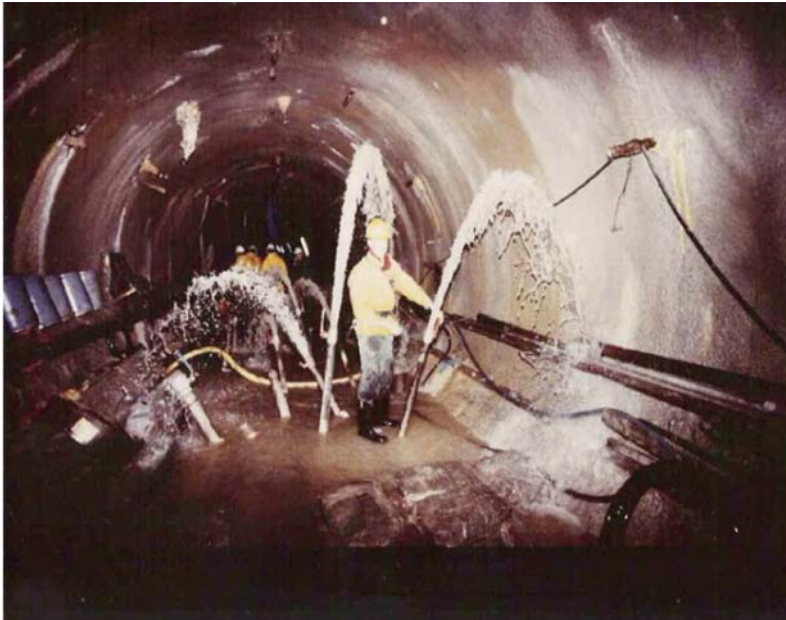
Fig. 4.10. Water inflows during LEP tunnel construction.
