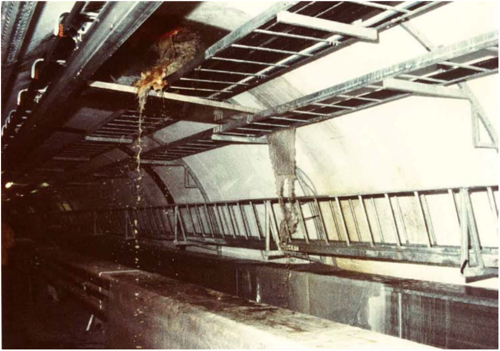
Fig. 4.11. Failure of tunnel concrete lining in 1990.
