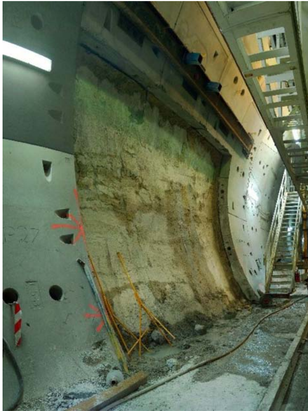
Fig. 4.6. An example of lining breakout from the Brisbane Airport Link, Australia (Arup).
